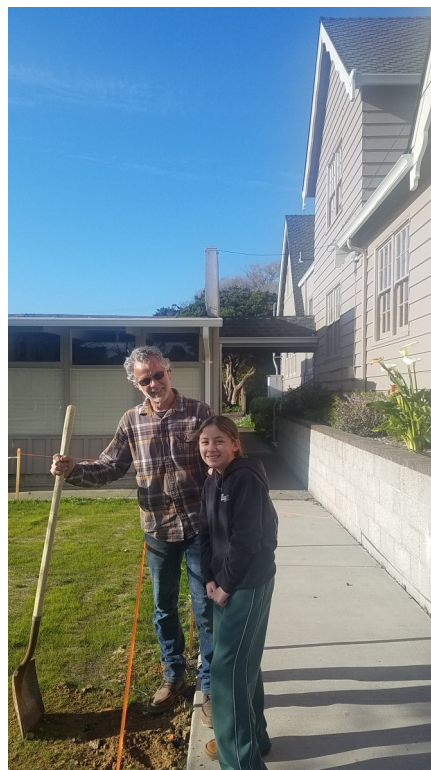
Dale and Grace installing sprinkler heads on McCarthy Meadow, future site of the labyrinth.
